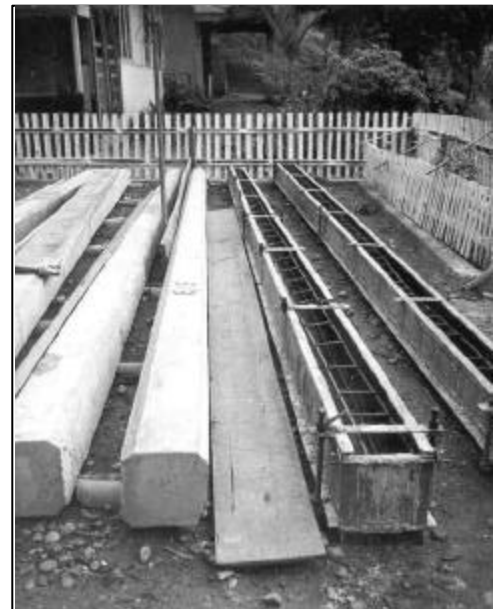
Fig. 11. Steel reinforcement placed in a mold ready for casting at an isolated site in Indonesia. Completed poles at the left are curing.
