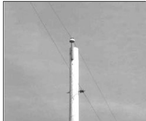
Figure 16. The simplicity of the poletop assembly associated with single-phase (phase-neutral) distribution is readily apparent.
