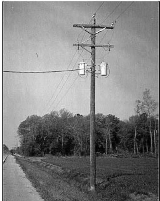
Figure 18. A two- or “vee”-phase line with two single-phase transformers providing three-phase power to workshop in eastern Maryland (United States).
