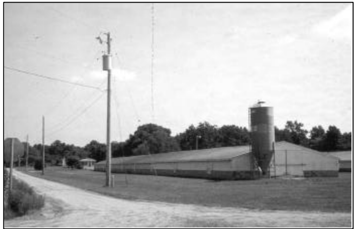
Figure 20. A 100-kVA single-phase pole-mounted transformer is adequate to serve the needs of this rural farm in the United States.
