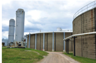
The City of Hamilton is upgrading its treatment plant to process higher flows and add tertiary treatment. Changes will result in more biogas generation in the digesters.
