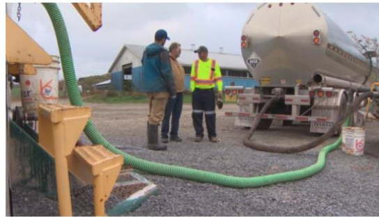
Courthouse Hill Energy in East Hants, N.S., is turning food waste into energy to sell to Nova Scotia Power. (CBC)
