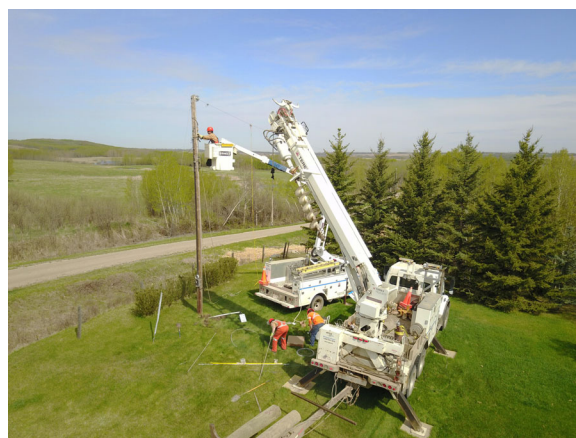
Electricity Distribution, Maintenance Work, Alberta
