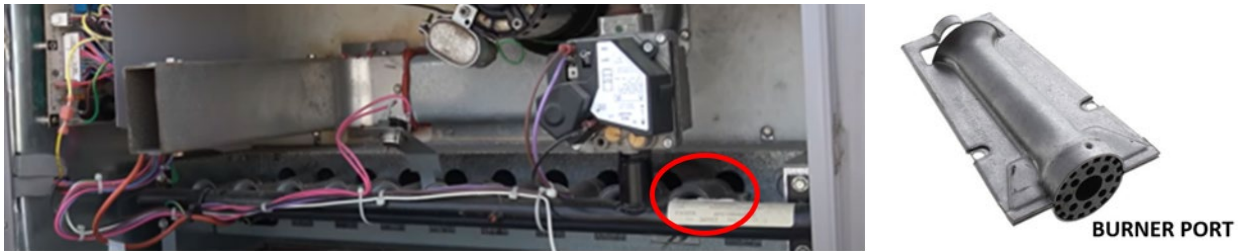
Figure 6-9: In-shot burner in roof top air conditioner (Left, red circle) and in-shot burner (Right)
